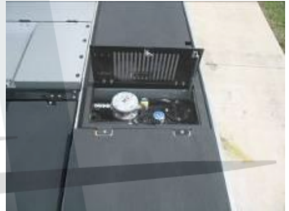
Hinged Cover to Hydraulic Tank Fill
