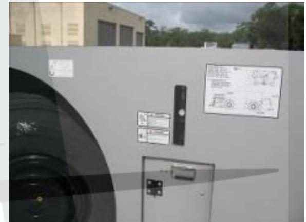
Recessed Hydraulic Level Gauge
